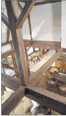
Handcrafted Homes' placement of beams in this Sandy Springs home signals where one room begins and another ends. CONTRIBUTED BY JOHN UMBERGER
